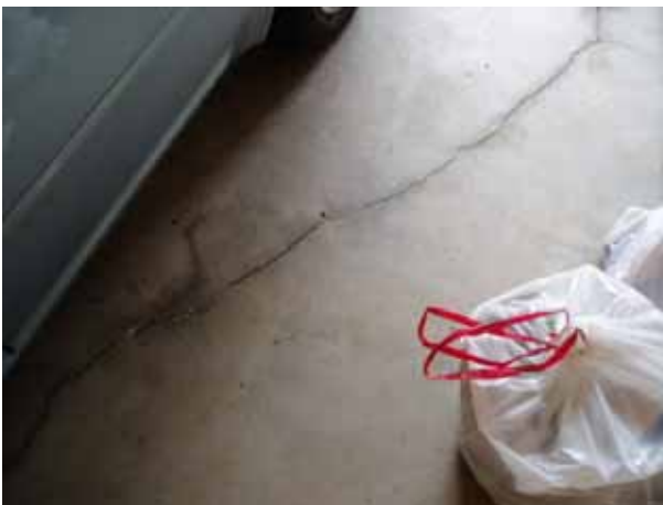
5. Cracks in concrete garage slab
