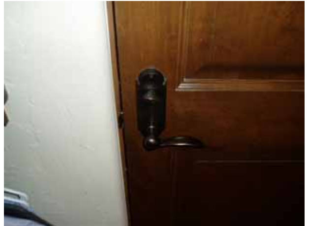
8. Dead bolt did not operate properly
