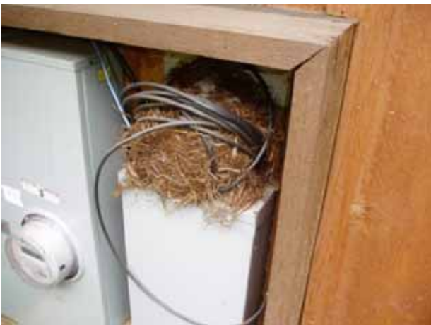
9. Animal nest in electric service entrance box
