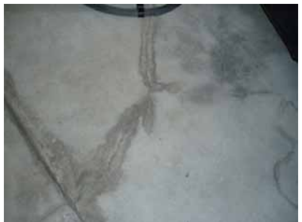
6. Cracks in concrete garage slab
