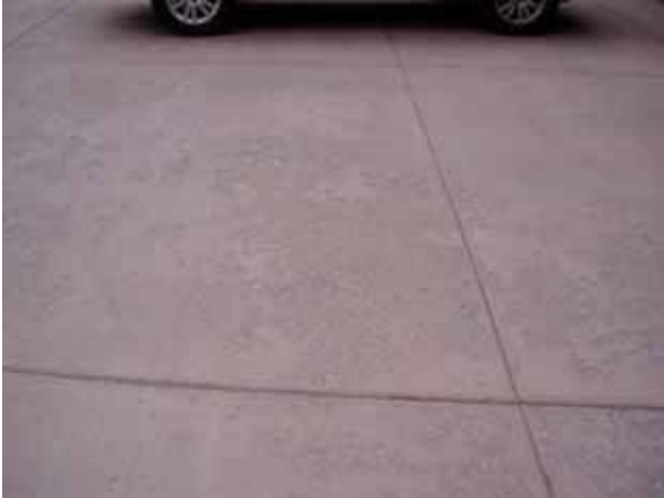
1. Spalling of concrete driveway
