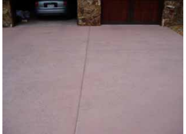
2. Spalling of concrete driveway
