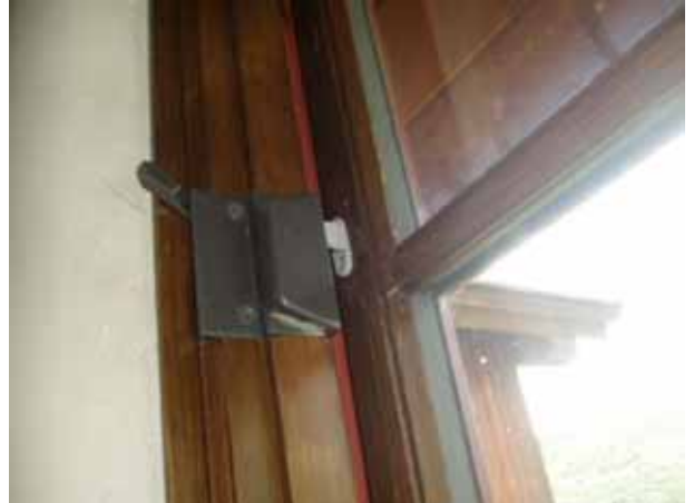
4. Window latch did not operate properly
