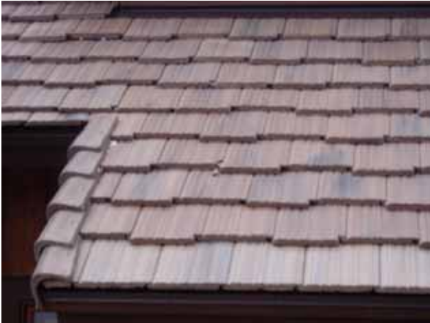
7. Small cracked piece of roof tile
