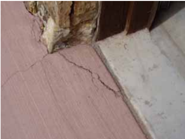
3. Crack in concrete driveway
